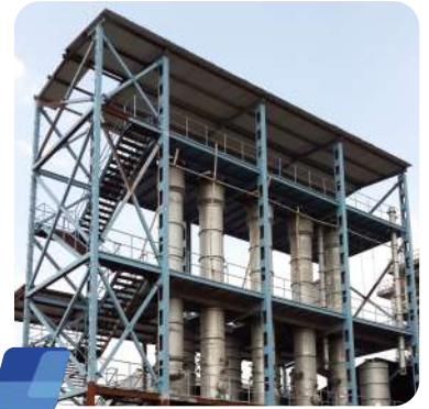
Waste Water Treatment System For ZLD
